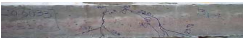
Figure 4. The formation of secondary cracks originating from the primary cracks leading to failure of beams without web reinforcing
