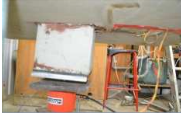
Fig 5 Punching of column in the flat slab after failure.
