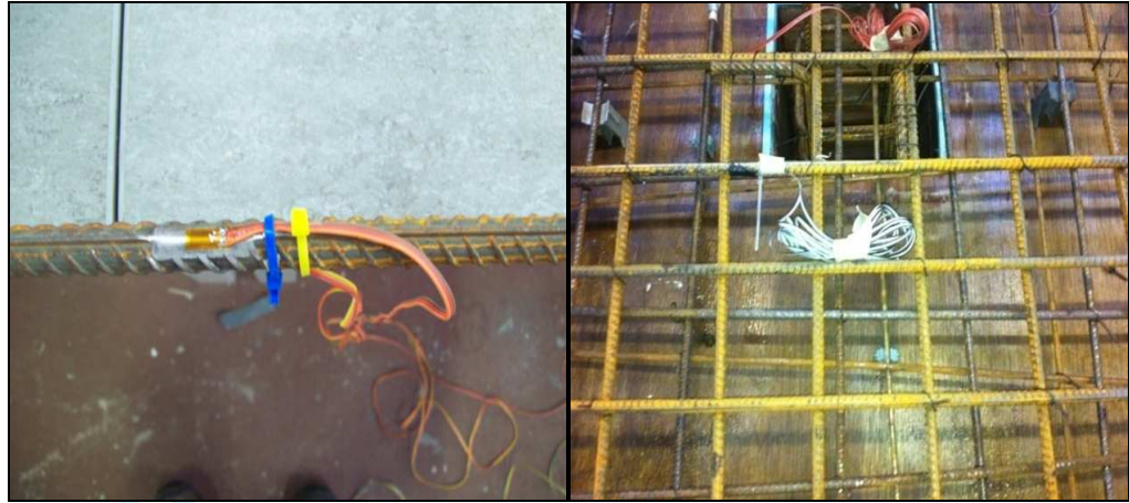
Fig 8 Location of strain gauges at tension bars near the face of column region
