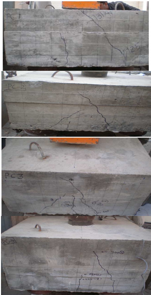
Figure 5. Failure modes of pile caps under external axial loads.
