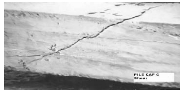
Fig. 6 Typical shear failure of pile cap
