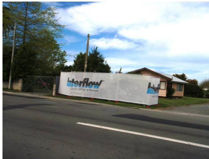
Figure 8. The footprint of the Rehabilitation of No.3 Trunk Sewer in Hastings, 628m of 1.8m diameter using Interflow's Rotoloc spiral wound lining technology.
